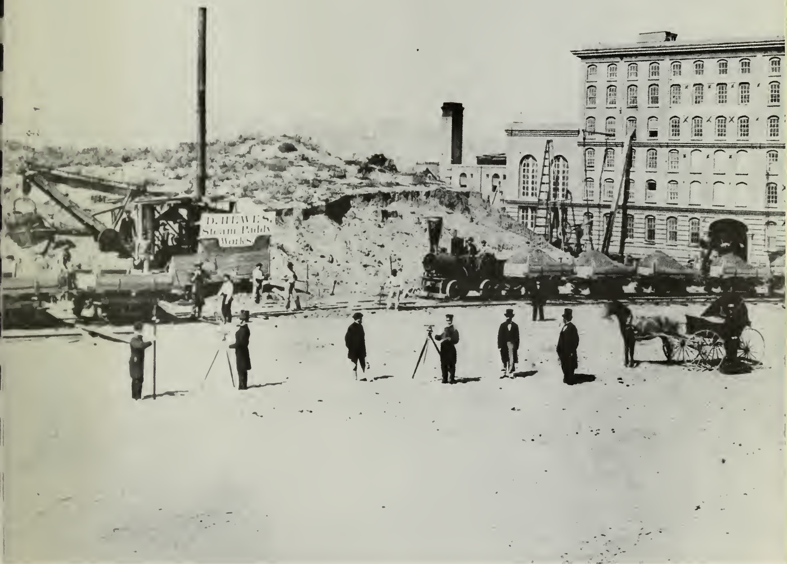
Plate 6: The Steam Paddy . . . D. Hewes, San Francisco's greatest practical leveler, poses with his workmen and associates in front of the steam shovel-and-dinky-train system that spread the sandhills north and south of market into Yerba Buena Cove and Mission Bay. This picture was made next to the sugar refinery at Eighth and Harrison in about 1868, some time after the steam paddy had done its work on part of the Yerba Buena Center. (Bancroft Library)
